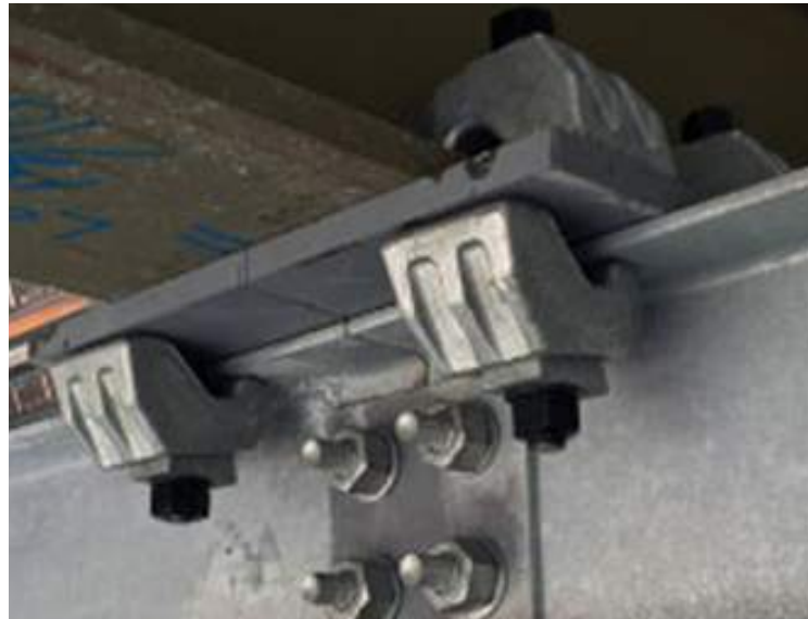
LINDAPTER CLAMPING SYSTEM AT AMERICAN COPPER BUILDING, SHOP ARCHITECTS
